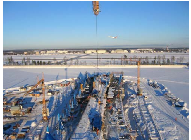
Construction continues around the clock on the New Terminal 3 at Moscow Shremetyevo Airport.
